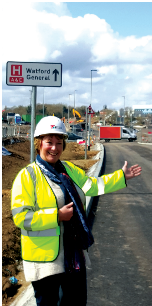
Providing a new access road helped to save acute hospital services in Watford.
