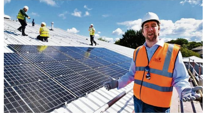
The Phoenix Centre in Newbury is one of six sites where solar panels are being installed with the help of local investment YOUTUBE
