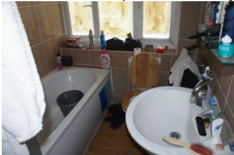
Photo 2: Bathroom shared by seven tenants, including four children
